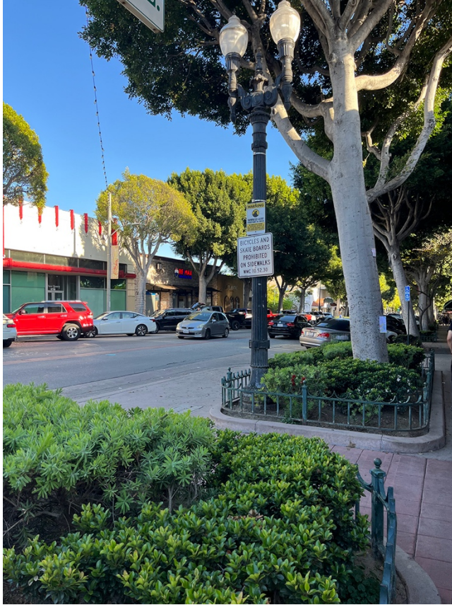
WHITTIER: Wrought iron barriers surrounding ficus trees on Greenleaf AV. These need to be refurbished and painted (picture taken April 27, 2024).
