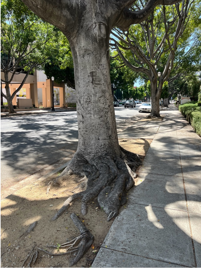
PASADENA: Ficus tree roots without surrounding barriers (picture taken April 27, 2024).
